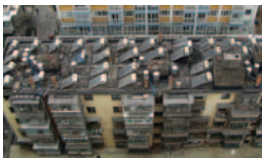
Photo 4.2 Solar water heaters in Kunming, China
