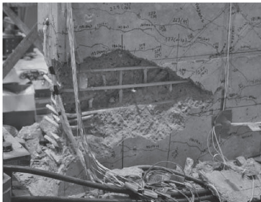
(b) Concrete crushing causing failure
