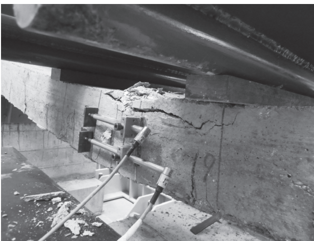
(b) Compression failure
