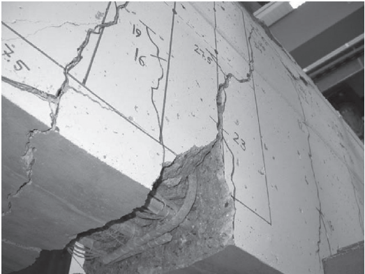
(b) Detail of failed concrete in compression and GFRP bar in tension
