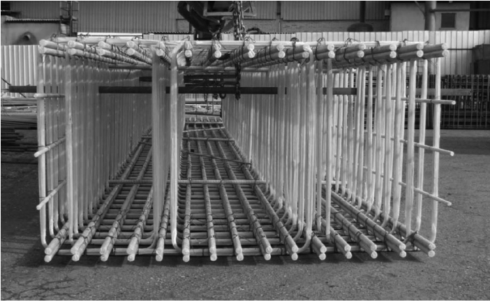
Figure 1.12 GFRP reinforcement cage for soft-eye construction at a manufacturing plant (Angri, Italy).
