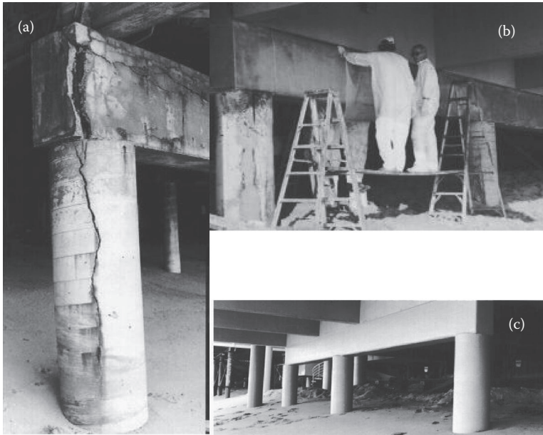
FIGURE 8.2 Damage caused by corrosion: (a) before repair, (b) after repair prior to strengthening, and (c) after strengthening. (Courtesy of Fyfe Inc.)
