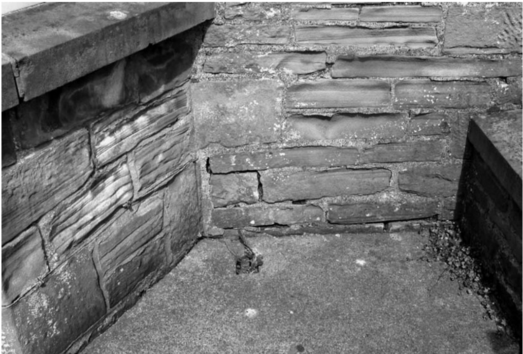
Figure 3.1: Damage caused by cement pointing.
