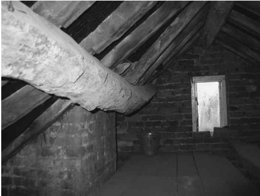
Figure 18.6: Photograph of a deflected purlin.
