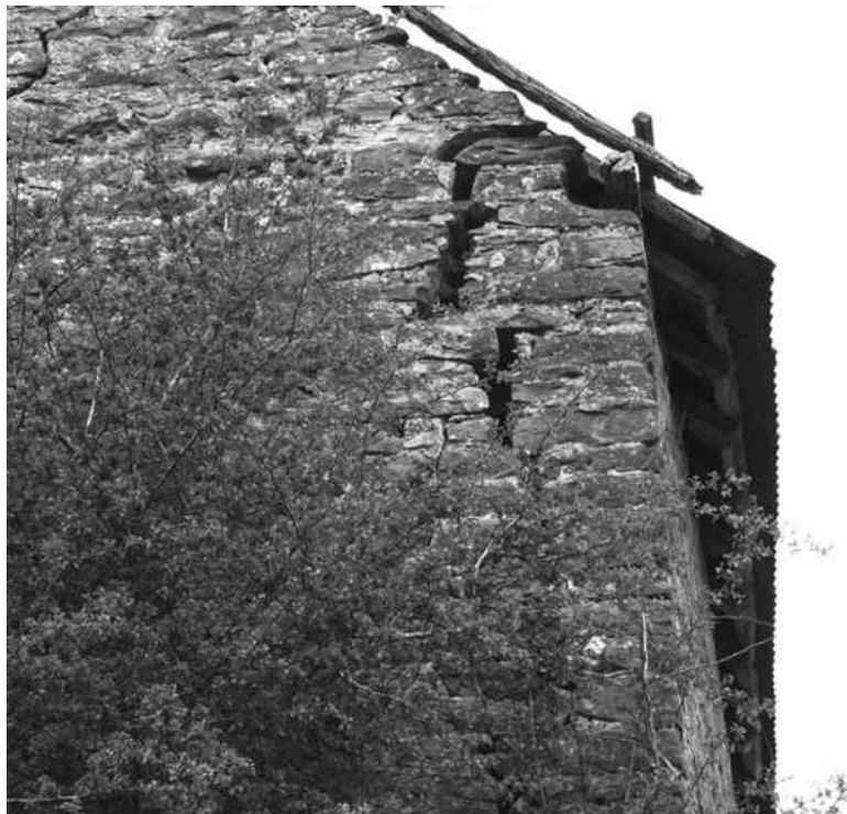
Figure 10.8: Photograph showing a property with roof spread.
