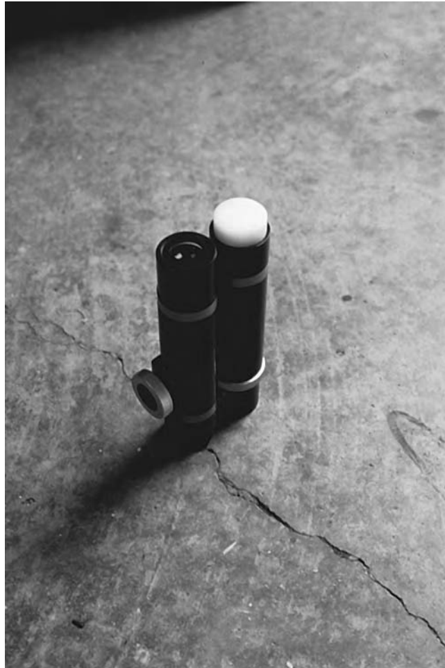
Figure 13.3 Measuring crack width with a 50x microscope
