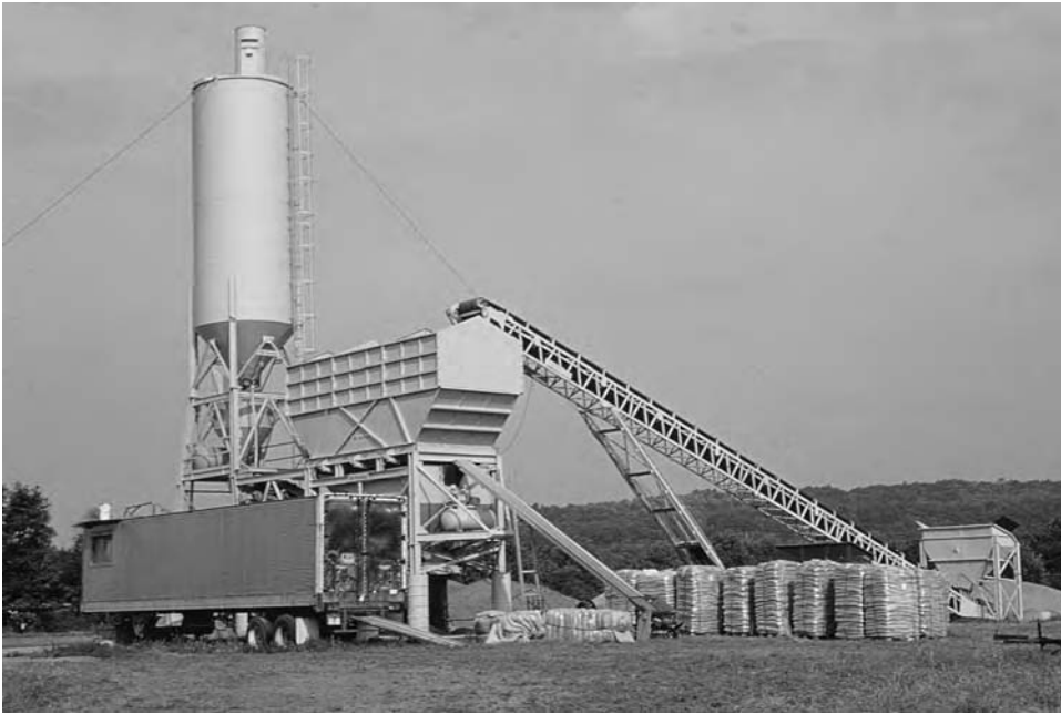
Figure 10.1 Temporary batch plant near the job site
