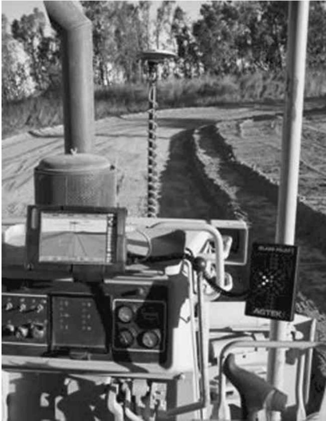
Fig. 9.28 GPS guided plant – courtesy of AGTEK Development
