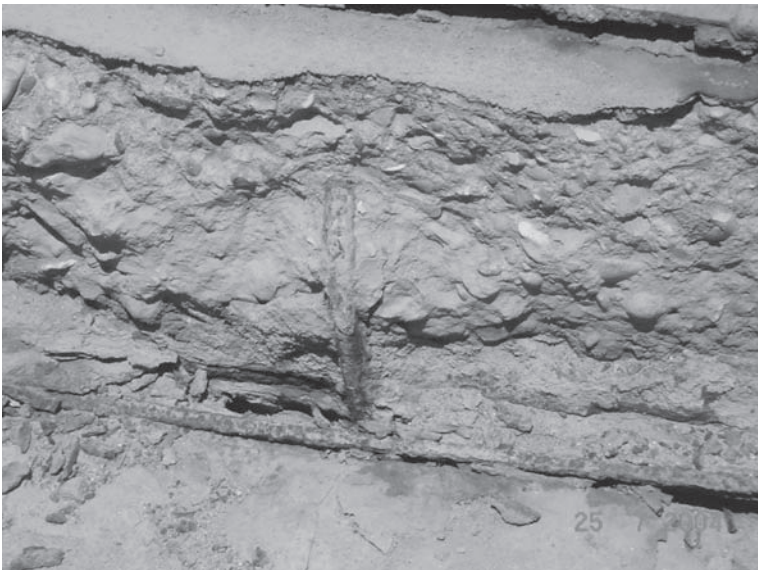
FIGURE 4.19d Reduction in steel cross-sectional area.
