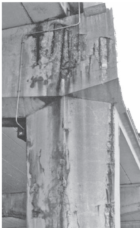
FIGURE 4.3 Brown spots on bridge column and girder.
