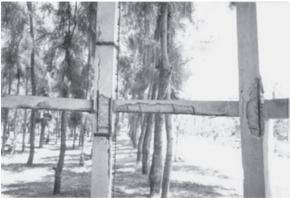
FIGURE 3.9 Photo of cracks on columns and beams.
