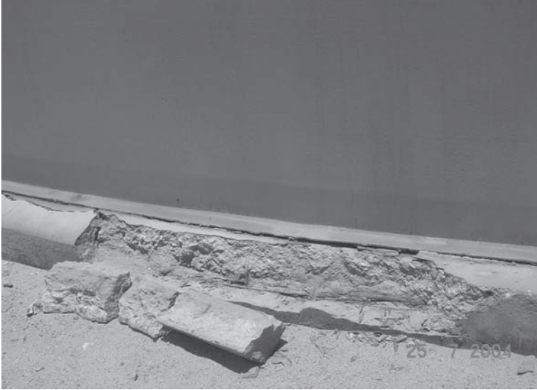
FIGURE 4.19c Spalling of the concrete cover.
