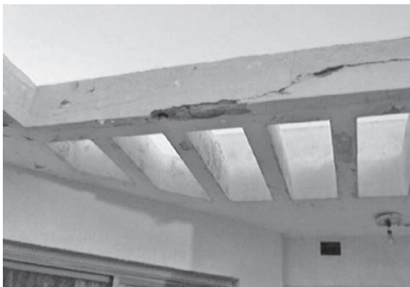
FIGURE 2.1 Deterioration in a reinforced concrete beam.
