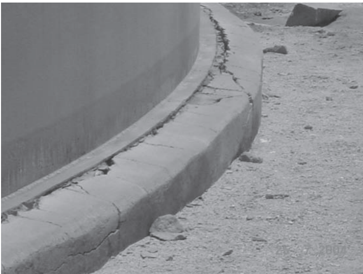
FIGURE 4.19b Cracks on the tank ring beam.
