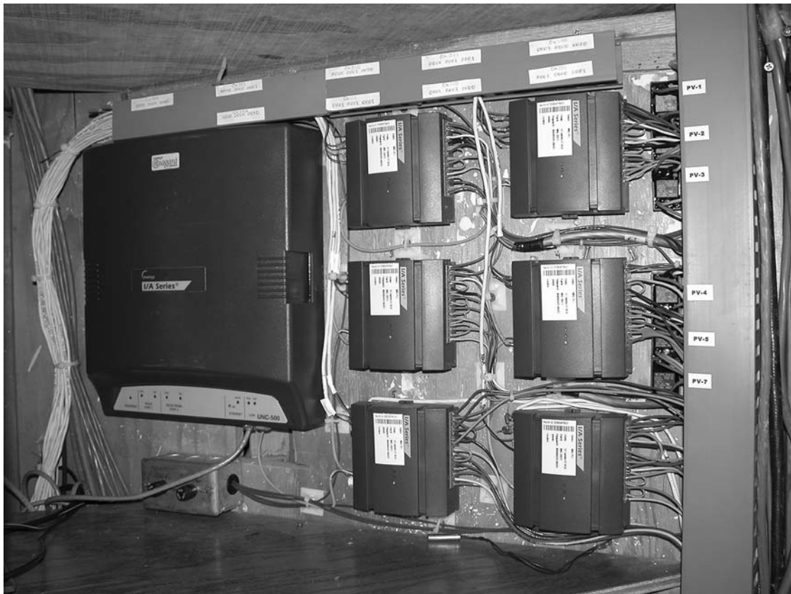
Figure 7.11 Photograph showing control closet hardware.
