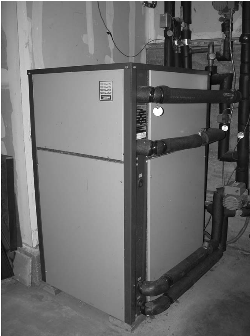
Figure 7.6 Photograph of Berkeley house geothermal heat pump.
